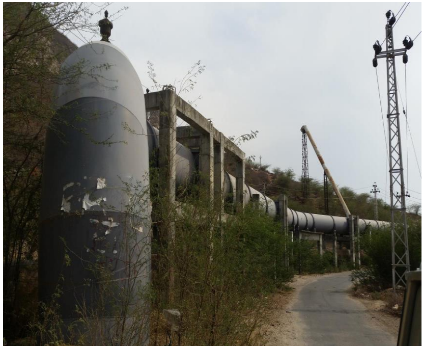
Figure 12. Exposed Pressurized Water Distribution Pipe
