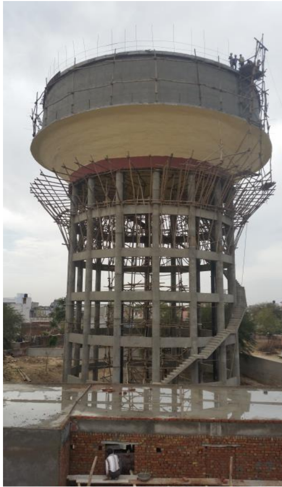
Figure 13. Gravity Pressure Distribution Reservoir
