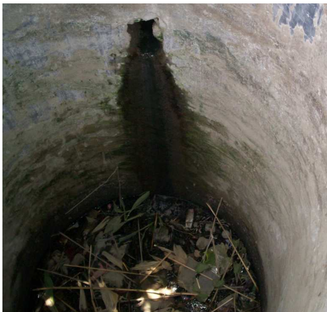
Photo 2: Domestic sewage being discharged directly into a well
