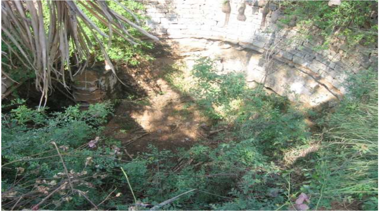
Fig 4: Dugwell-Totally Failed in Non-JFPM Area
