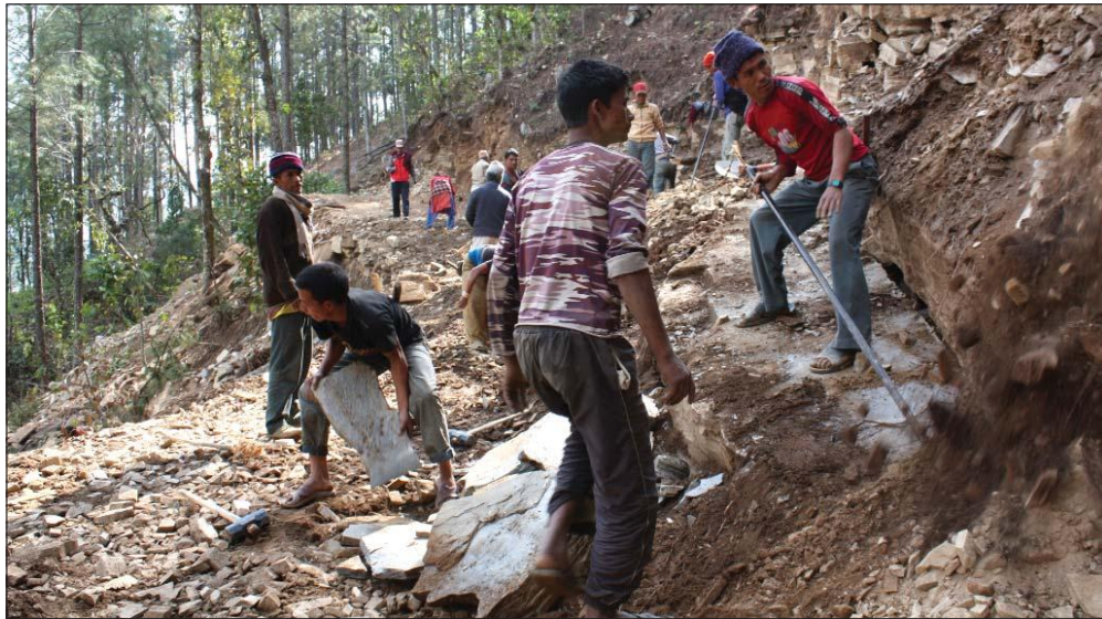
Local people participating in rural agriculture road construction in Naumule VDC, Dailekh
