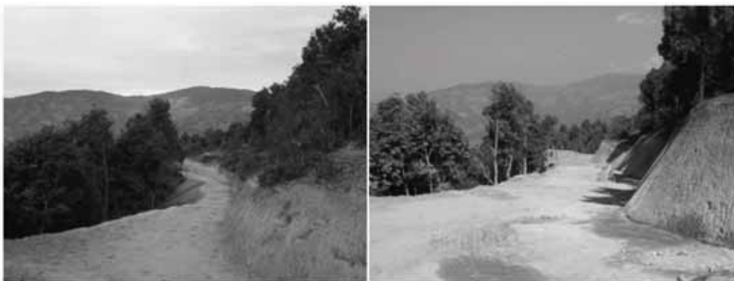
Figure 7. Phase construction; first phase 2.5m track opening to gradual widening to 4.5m road length. (Source: Dhakal IS, 2007)
